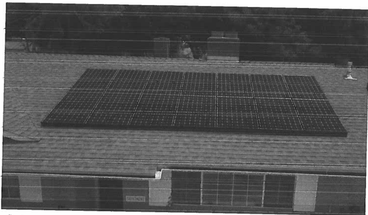
SunPower is providing the solar panels for the Menifee microgrid housing development. (Photo courtesy of SunPower)
