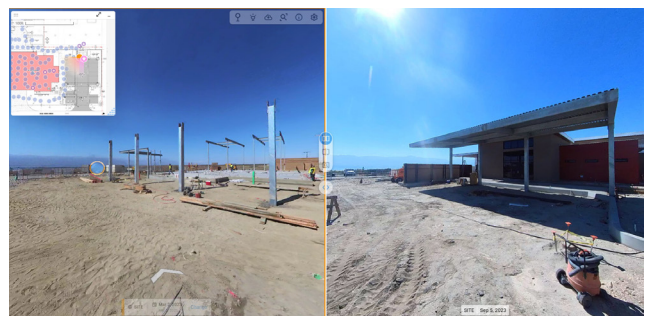
Pictured (Fire Station 41, Mecca): Example of 360 degree virtual project walkthrough compared by timeline (March 2023 and September 2023)
