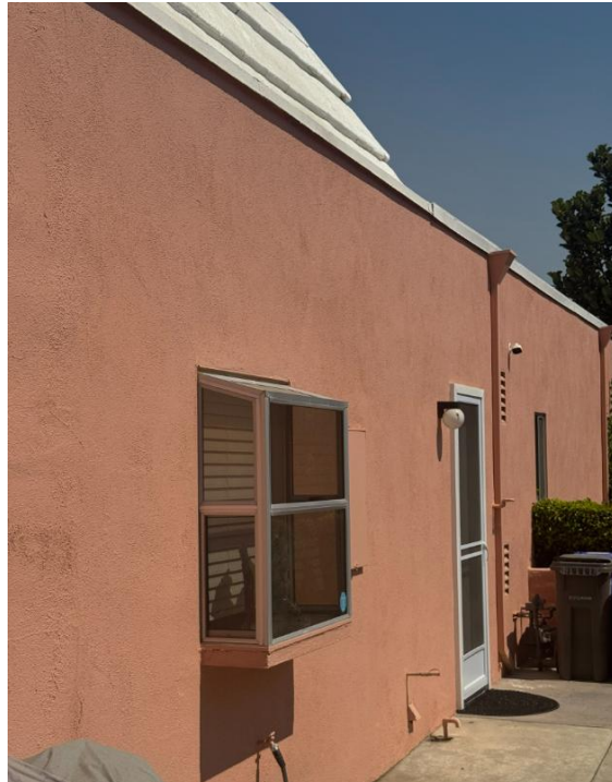
Figure 1 – Non-original window type in original opening
