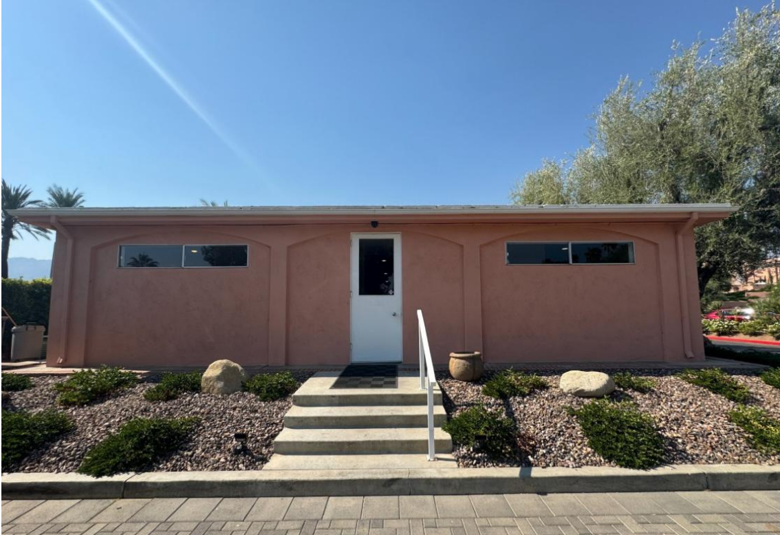
Figure 5 – Non-original windows and door of administrative building set within original building recesses
