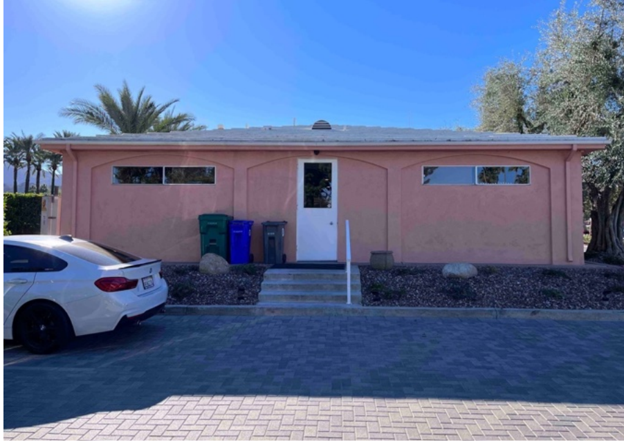
The rear (north) elevation is a symmetrical design with a single door and two symmetrical windows. The original archways are also expressed in the stucco of the walls. Rear (north) elevation, view south.
