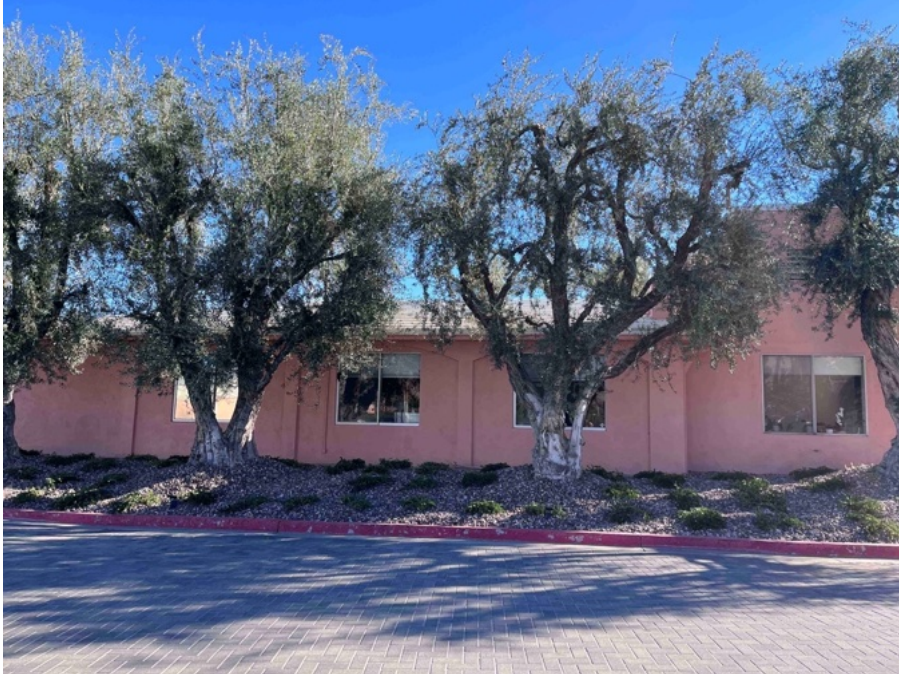
The side (west) elevation of the Administration Building shows the transition between the shed roof and the hip roof. Running down the side of the building is a set of windows set within archways expressed in the stucco. Side (west) elevation, view east.
