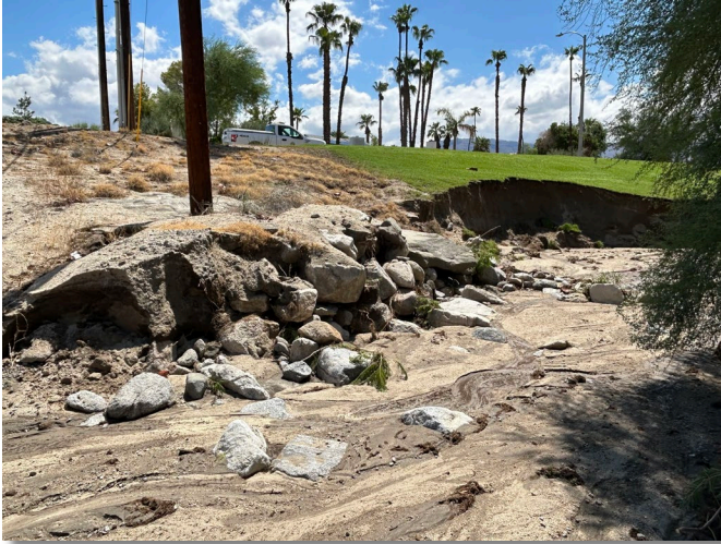
Looking South: SCE Power Pole
