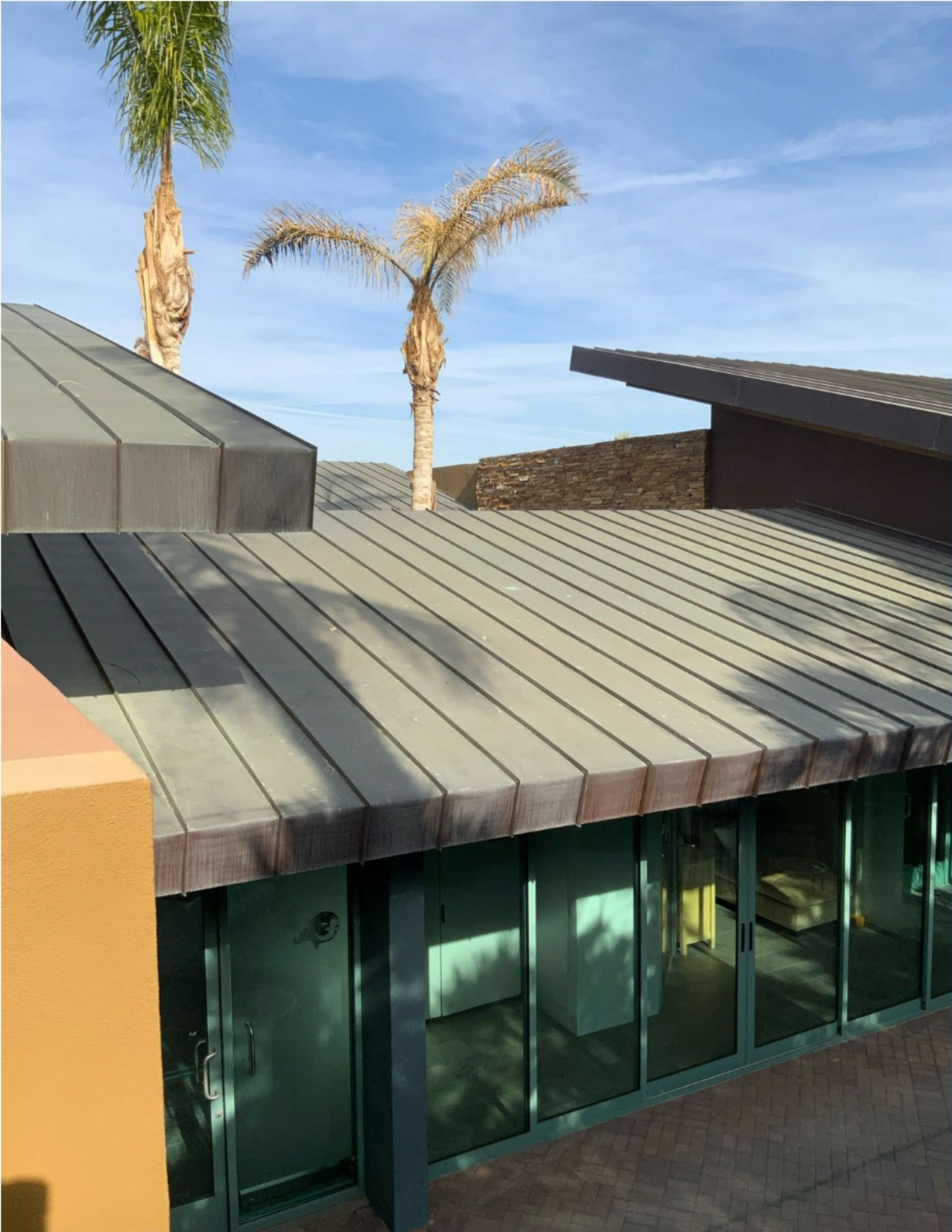
Rear roof at building infill part of atrium enclosing and new treatment rooms 6 & 7
