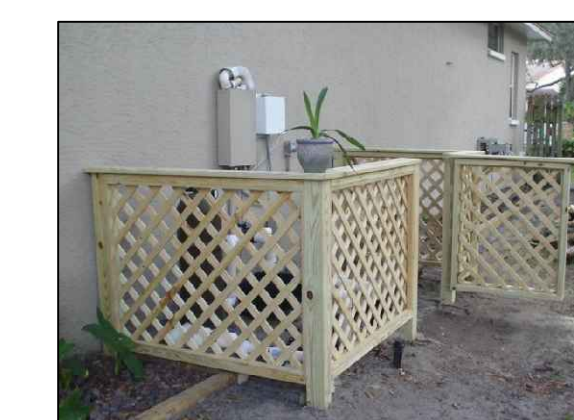
GAS METER SCREEN
